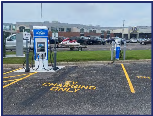
Figure 15. EV Charging Stations
