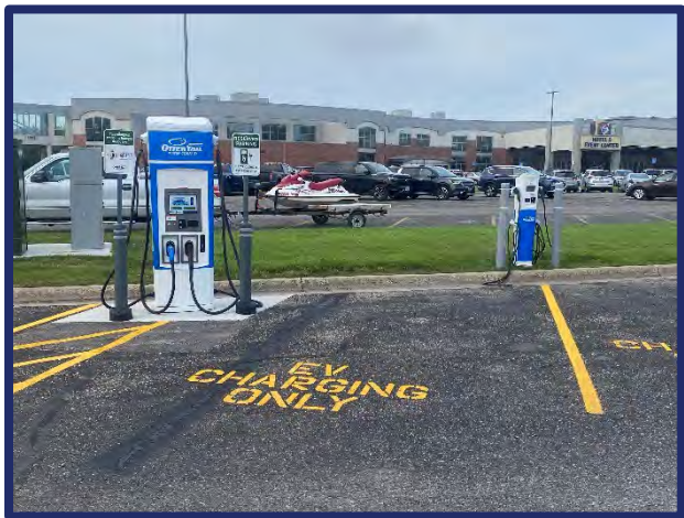
Figure 13. EV Charging Stations
